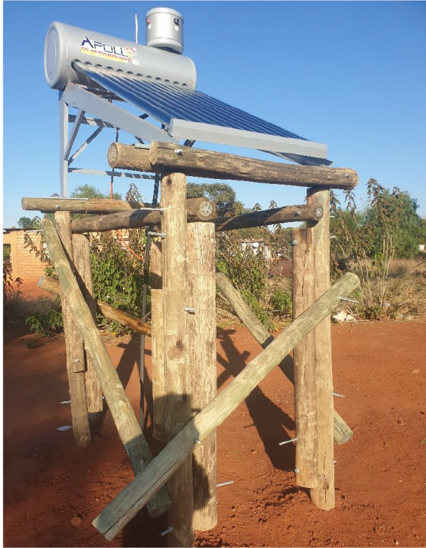
Figure 27: Solar water heater
