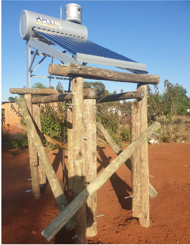
Figure 27: Solar water heater
