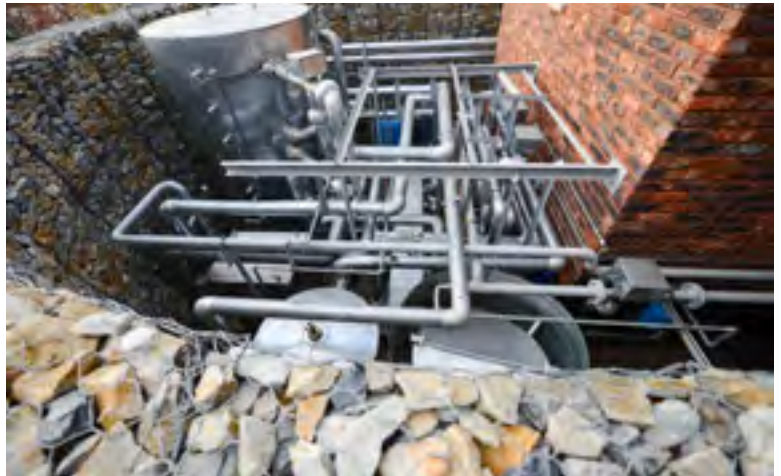
Above: Vodafone Site Solution Innovation Centre (SSIC) Cooling Plant, Midrand, 2011. GLH Archive.
